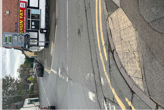
Figure 7 Disrepair of surfaces create an unpleasant walking environment
